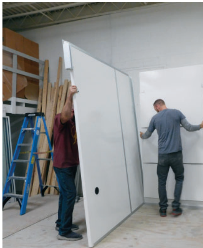
Attach Panel (Left Side Wall A) to (Left Side Back Wall B).
