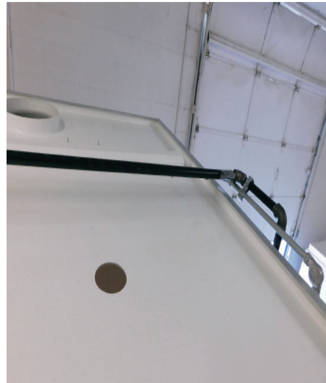
Fire Suppression System from top of hood
