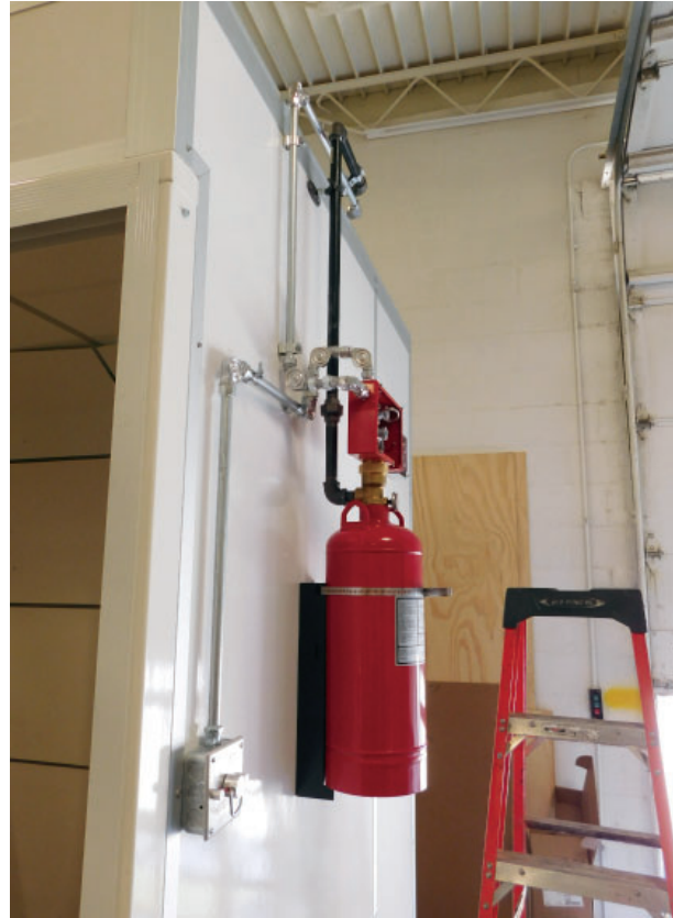
Fire Suppression System
