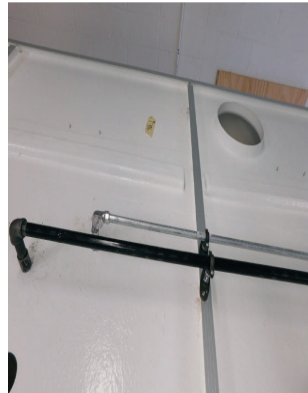
Fire Suppression System from top of hood
